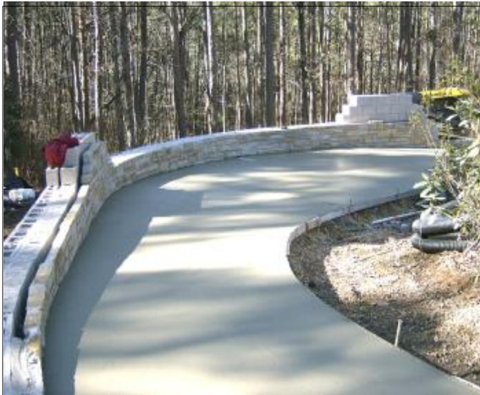
A wide and gently sloping handicapped-accessible walkway was recently completed at the columbarium site.
